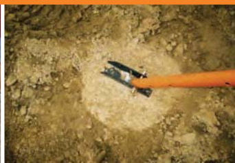
Same brackets attach at anchor location
