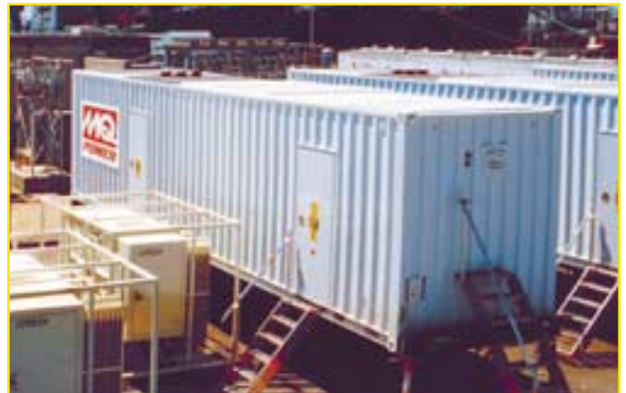
Containerized Generator (EGC-1500C)
